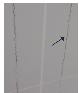
Cracks formed in PA backsheet after four years of field exposure
