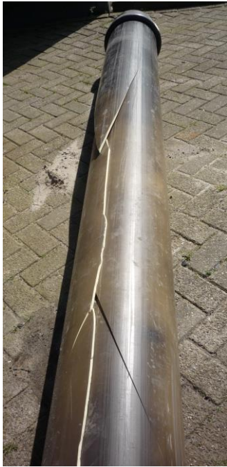
Figure 1. PVC water pipe after RCP. The crack initiated in the middle and ran in two opposite directions. Both branches show bi- or tri-furcation.
