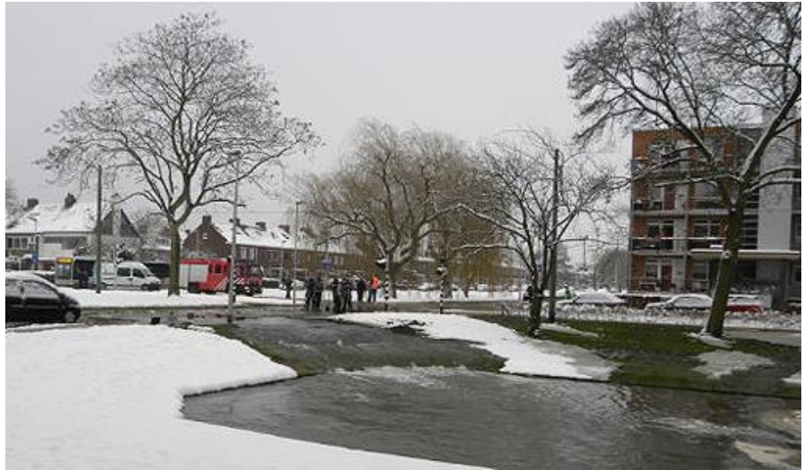
Figure 2. Water flows through the snow after RCP in a PVC water pipe.
